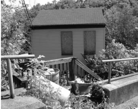
ABOVE: Garbage and debris are obscuring this vacant hilltop house. Photo by Paula Martinac
