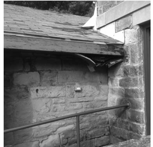
ABOVE: The roof of the historic arsenal's magazine is rotting and falling off. Photo by Jill Harkins
