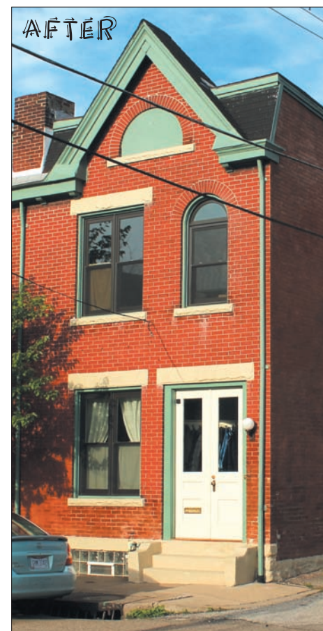
ABOVE: After the facade grants came through, the owner of this Garfield home was able to re-point the brick, install a new door, and put down a new paint job. Photo by Keith Williams.
